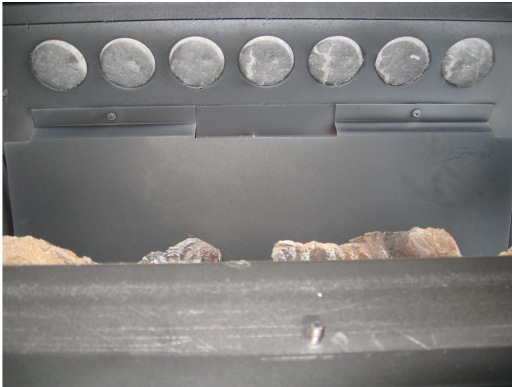
Pressure Relief Openings on Top of Firebox
